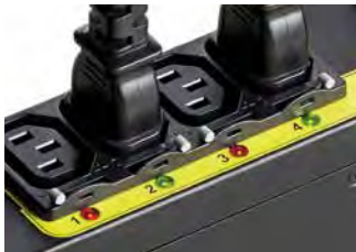
Green LED signifies power on and red is power off to outlet
